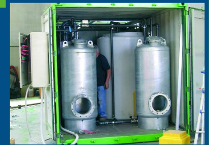
Containerized WWTP - 50 m 3 /d drilling rig camp Saudi Arabia
