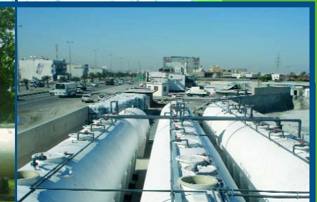
WWTP - 300 m 3 /d construction camp Bahrain
