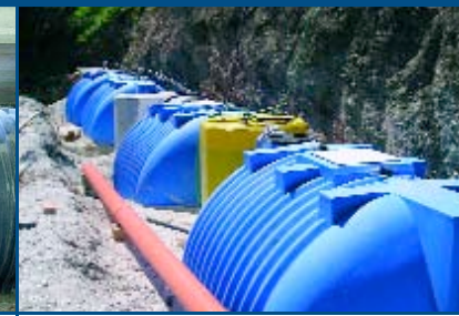
WWTP - 40 m 3 /d discotheque Italy
