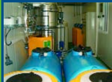
Food processing wastewater treatment plant Italy
